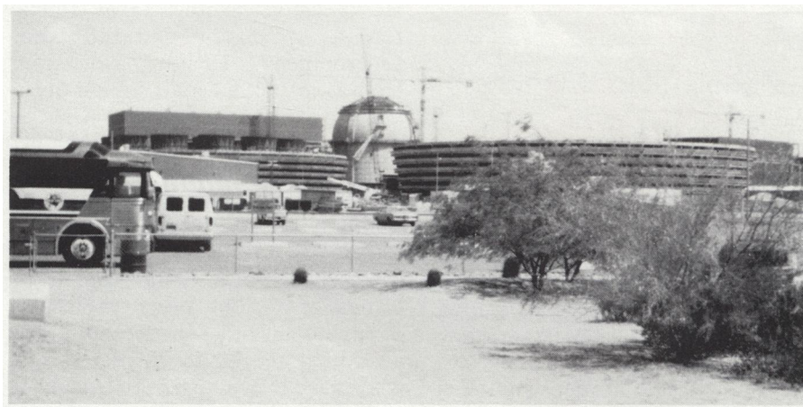
Nuclear power plant under construction near Phoenix was visited by early conference goers.
